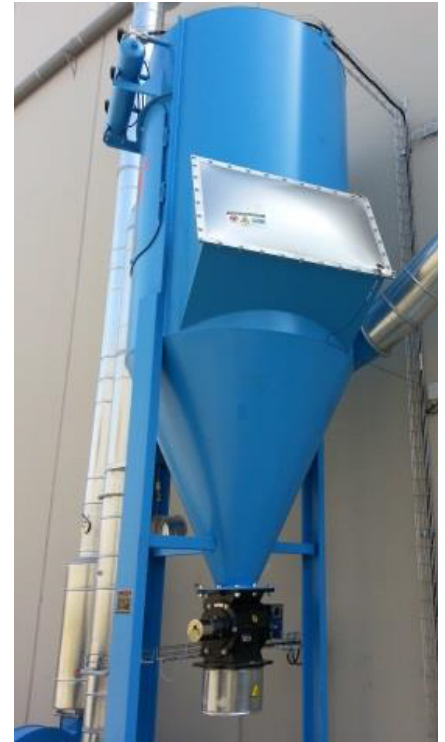
Vent panel on cyclone filter
